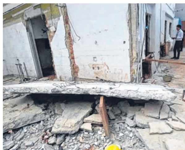
The fallen balcony slab, which trapped a worker beneath it in the incident at a house reconstruction project site in Hougang in 2019. The worker was pronounced dead at the scene, while another worker was injured. PHOTO: MINISTRY OF MANPOWER
